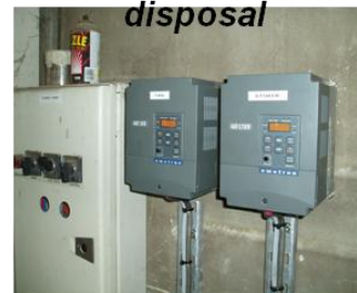
VSD controls for auger and fan
